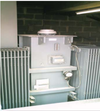
Project: PSU Project: CTRL 104H MML Sub-Station
